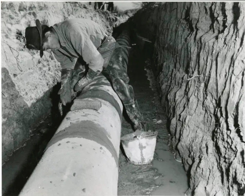
A member of a CCC-ID crew cementing the joints in a pipe line built on Santa Clara Pueblo lands for diverting irrigation and drinking water to the pueblo lands and surrounding areas. December 1940. Photo: W.J. Mead, National Archives, ID: 35-G-17C-2077.
